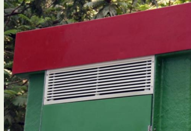
Louvers at top position of the shelter
