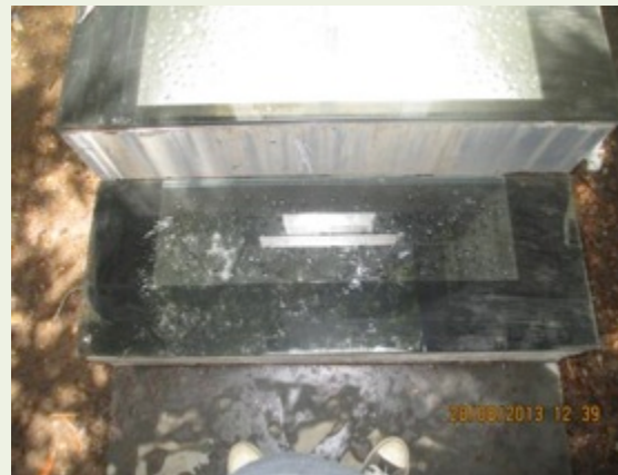
Glass window to monitor solids pit
