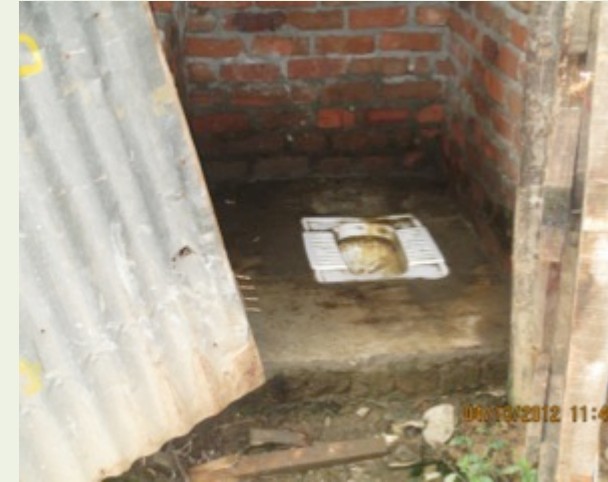
Contractor Labour colony toilet, IITB
