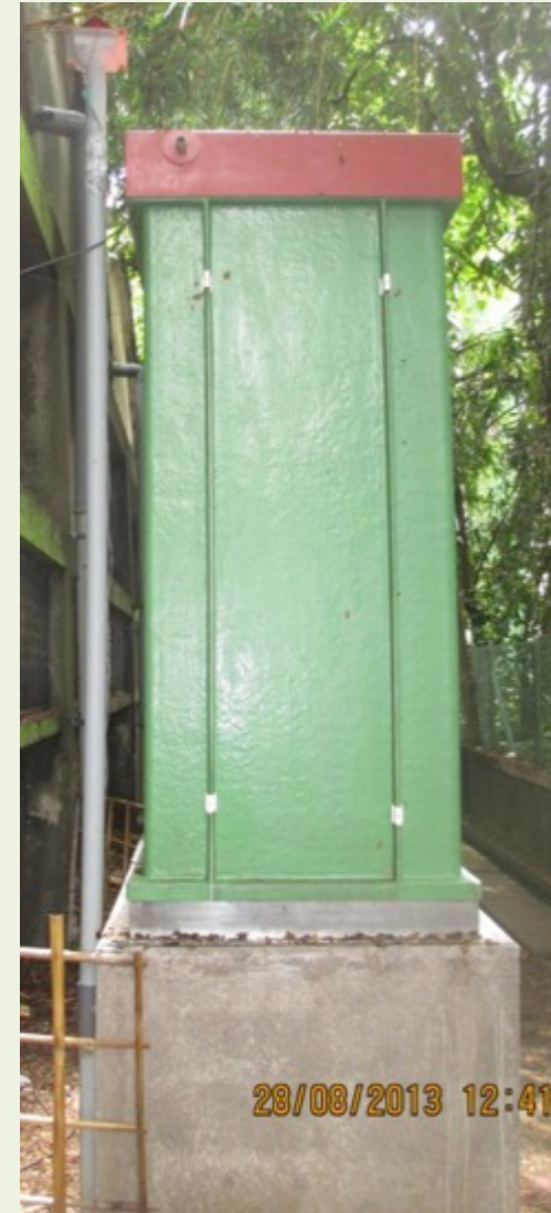
Vent pipe for solids pit
